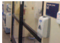
Automatic isolation room door with "knowing act" touchless system to ensure doors are only opened when activated
